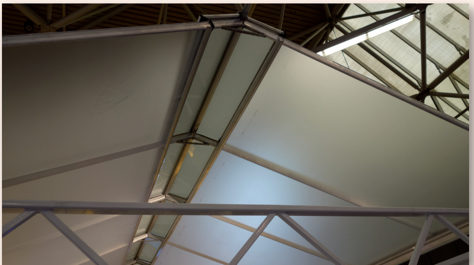
Greenhouse structure fitted with ETFE film beneath glass as seen at Greentech 2016
